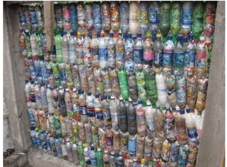
Bottles strung to chicken wire on one side. Now the chicken wire will be placed on this side as well. flickr.com
