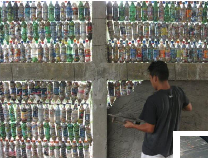
Neater job = better trowel... This is the 5th Hug it Forward school, under construction in La Cereza, finished July 2010. hugitforward.com
