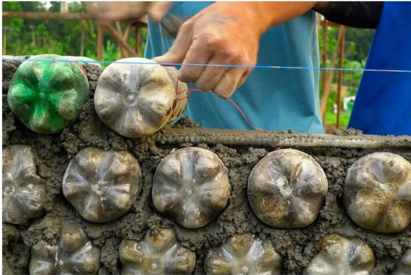
String is used to keep the bottles in place as the adobe is being applied.
